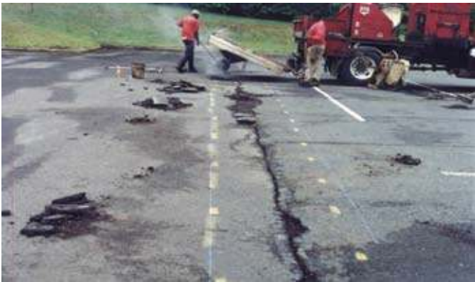
Severe parking lot crack (before)
